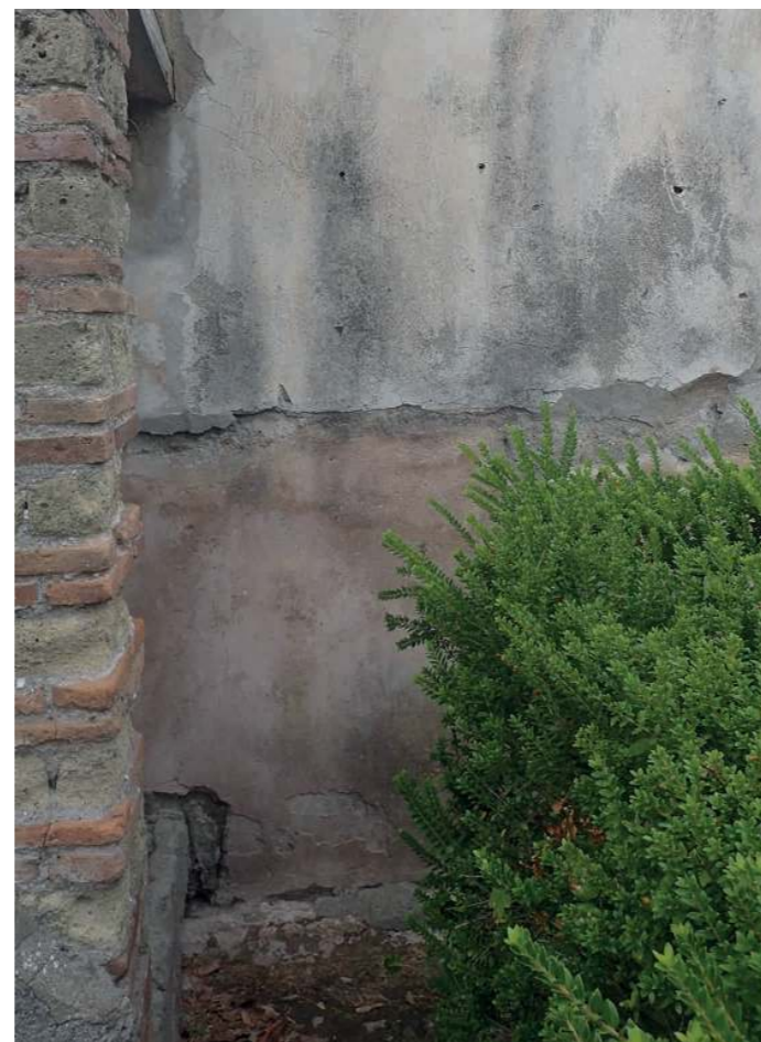
Fig. 3A. A wall in the garden of the House of the Deer showing the distinct change in decoration from the cocciopesto lining at the top
