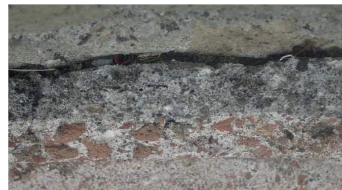
Fig. 1. The two distinct layers of the waterproof linings in Herculaneum: a bottom preparatory layer with volcanic aggregate and top water interfacing layer with crushed terracotta aggregate.
